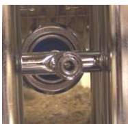
No water valve in place
